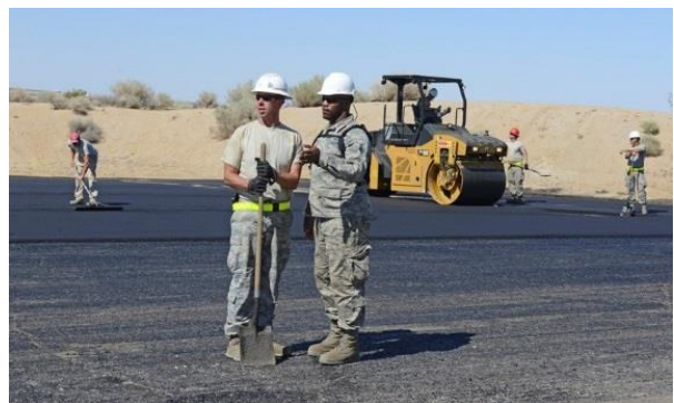
Civil engineer Airmen lay asphalt in front of Club Muroc as part of a complete repaving project. More than 80 Airmen from across the nation joined 412th Civil Engineer Squadron personnel to complete three large construction projects at Edwards.
