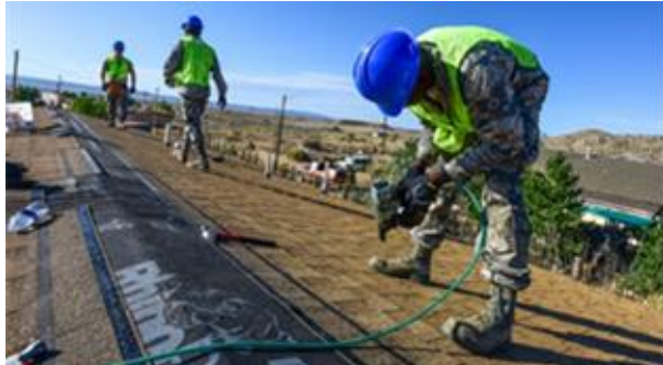
U.S. Air Force Staff Sgt. Cormick Blueford, an electrical technician assigned to the 169th CES, nails shingles to the roof of a home for a Native American veteran.
