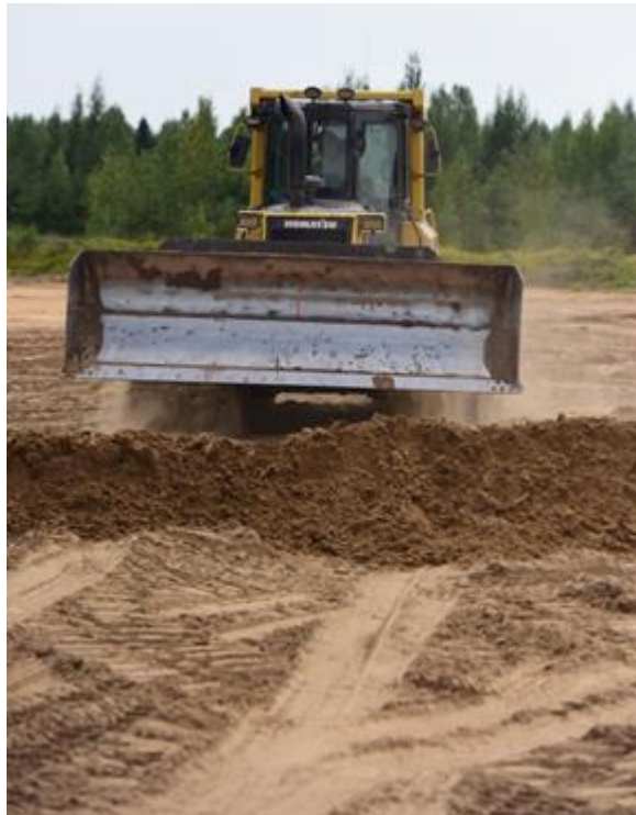
Tech. Sgt. Jacob Wallace, airfields' team lead with the 201st RHS Engineers, operates a bulldozer to clear the ground in the process of creating a military air-to-ground training range. The range will include a mock village, bomb circle, simulated runway, fire break, strafe pit and an observation point.
