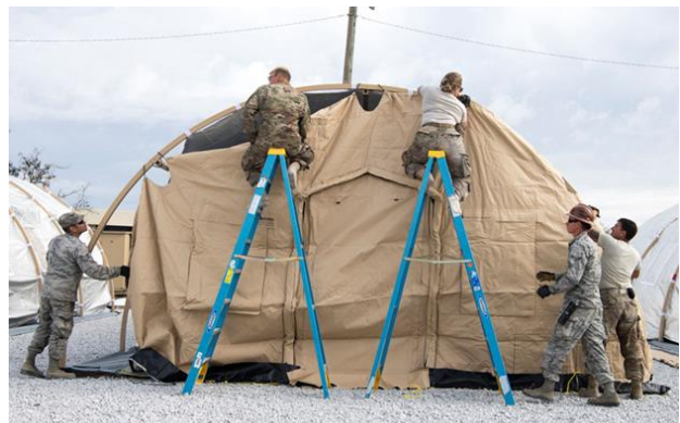
Airmen from the 23rd Civil Engineering Squadron, Moody Air Force Base, Ga., and the 635th Material Maintenance Squadron, Holloman AFB, N.M., add to the dozens of housing tents they have helped construct on Tyndall AFB, FL., October 25, 2018.
