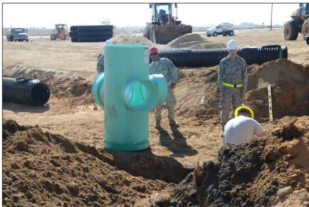
Civil engineer Airmen with the help of 412th CE Squadron personnel install an underground drainage system near Kincheloe Ave near base housing.
