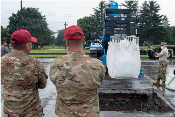
Training cadre from the 554 th RED HORSE Squadron out of Andersen Air Force Base, Guam, oversees a civil engineer Airman position equipment prior to backfilling a crater while conducting Rapid Airfield Damage Repair (RADR) during Pacific Unity 2019.
