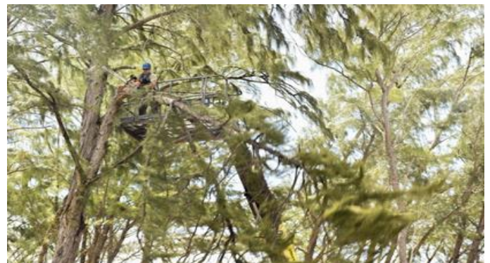
U.S. Air Force Staff Sgt. Bradley Moore, a heavy equipment operator assigned to the South Carolina Air National Guard’s 169 th Civil Engineer Squadron, uses a chainsaw to cut down an aged and invasive ironwood tree at Bellows.
