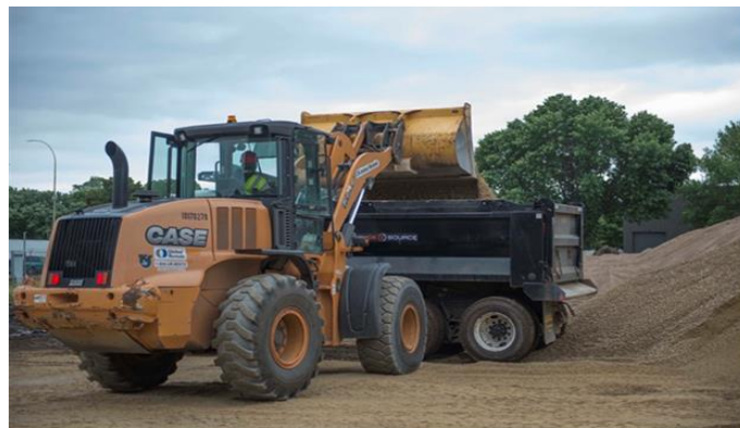
Master Sgt. Johnny Cunningham, 560 th RED HORSE Squadron rotational NCO in charge, pours material into a 20-ton dump truck using a front end loader at a construction site on Minneapolis-St. Paul Air Reserve Station, Minn., July 10, 2019. (U.S. Air Force photo by Tech. Sgt. Amber E. N. Kurka/Released)
