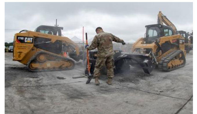
Senior Airman Tyler Crisp, 8 th Civil Engineer Squadron electrical systems journeyman out of Kunsan Air Base, Republic of Korea, motions to a heavy equipment operator while conducting RDAR during Pacific Unity 2019 at Yokota Air Base, Japan, August 22, 2019.
