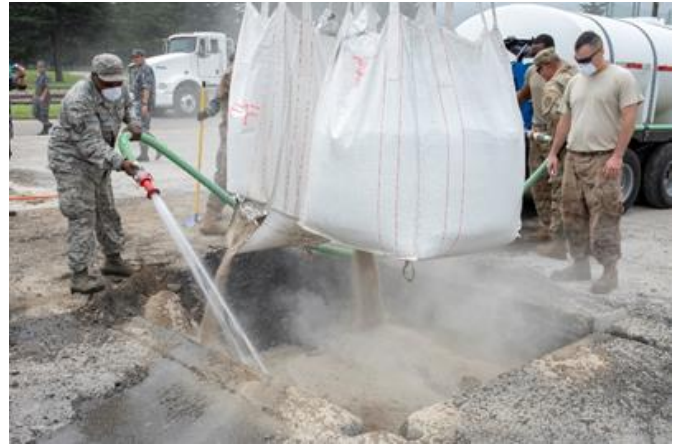
Civil Engineer Airmen mix water with flowable fill rapid set concrete to complete the backfill portion of RADR).
