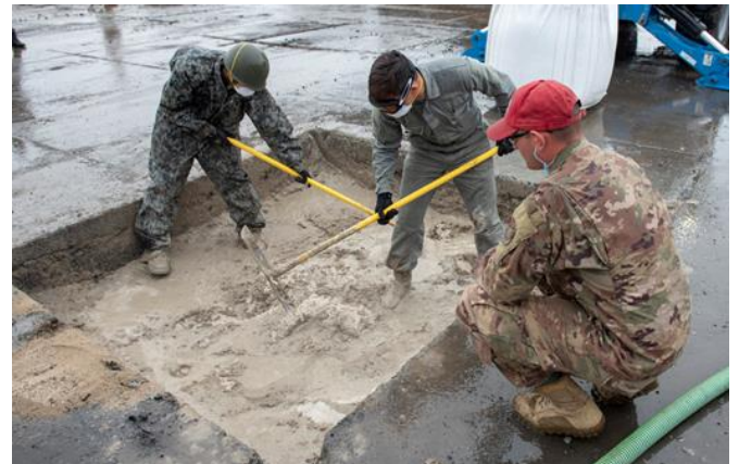
Training cadre from the 554 th RED HORSE Squadron out of Andersen Air Force Base, Guam, oversees U.S. Air Force and Japanese Air Self-Defense Force civil engineers mix water and flowable fill rapid set concrete to complete the backfill portion of RADR.
