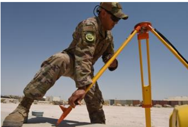
Senior Airman Javier Rodriguez, 379 th Expeditionary Civil Engineer Squadron geo-base technician, sets up a tripod to help him map an area for a new structure at Al Udeid Air Base, Qatar.
