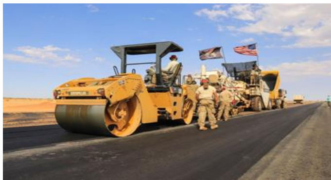
Airmen from the 31 st Expeditionary Squadron use a steamroller to compact and level asphalt while paving a flight line on Nigerien Air Base 201, Niger, in December 2018. (Additional story and photos by John Vandiver, Stars and Stripes, published May 22, 2019.
