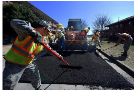
LITTLE ROCK AFB, AR. Sr. Airman Allen Arceo, a pavement and heavy equipment craftsman with the 19th CES, uses a "lute tool" to spread the asphalt evenly. (Photo by Airman 1st Class Kevin Sommer Giron)
