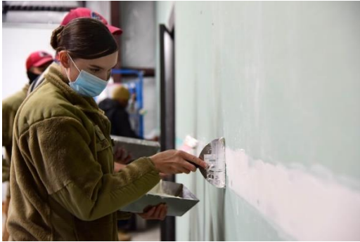
U.S. Air Force Sr. Airman Savannah Smith, a 554th RED HORSE structures journeyman, applies joint compound to a building partition at Eielson Air Force Base, Alaska, Sept. 10, 2020. The 554th RED HORSE Squadron specializes in large-scale construction projects including airfields, facilities and aprons.
