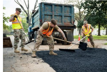
BARKSDALE AFB, LA. Sr. Airman Jacob Bishop (center), 2nd CES pavement and equipment journeyman, spreads asphalt. (U.S. AF photo by Sr. Airman Lillian Miller)
