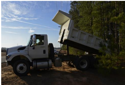
SHAW AFB, SC. U.S. Air Force Sr. Airman Joshua Minton, a pavement and construction equipment apprentice with the "Dirt Boyz" of the 20th CES unit, works on a beautification project. (Photo by Airman 1st Class BrieAnna Stillman)
