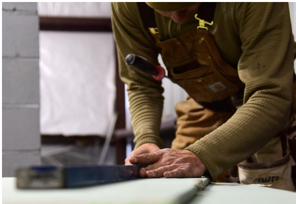
U.S. Air Force Staff Sgt. James Ori, a 554th RED HORSE structural craftsman, cuts off a piece of drywall at Eielson Air Force Base, Alaska, Sept. 10, 2020. The 554th RED HORSE squadron is comprised of Airmen from various Air Force Specialty Codes allowing it to be a self-contained unit capable of operating in contested environments.
