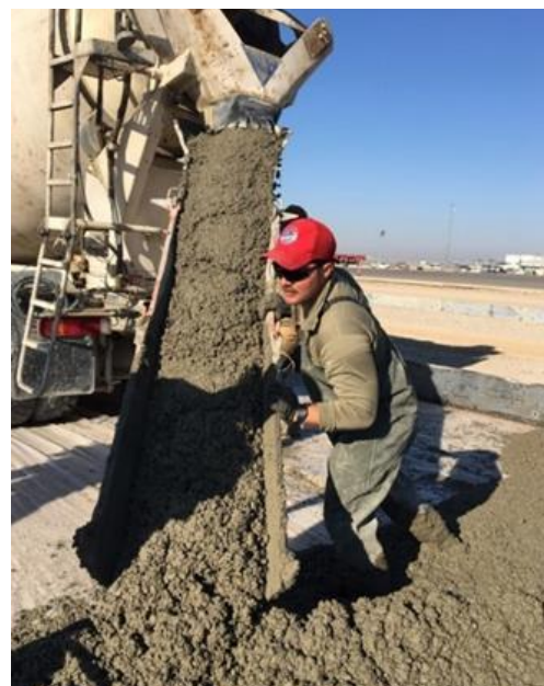
SSgt Bradley Wanner, an Airfields Journeyman assigned to the 557th Expeditionary Red Horse Squadron, guides the placement of concrete during the construction of the airfield parking apron located on Erbil Air Base, Iraq, on 04 November 2019.
