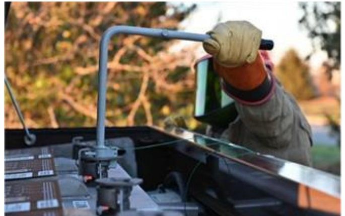
Senior Airman Taylor Tritten, 87th Civil Engineering Squadron electrical systems journeyman, operates a switchgear and shuts down power to a generator as part of the ERRE training.
