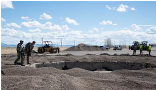
Inspecting a crater after a simulated mortar attack which involved assessing and repairing damage that could be caused during contingency operations.
