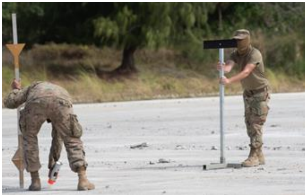
Airmen with the 554th RED HORSE Squadron prep an Airfield for repair.
