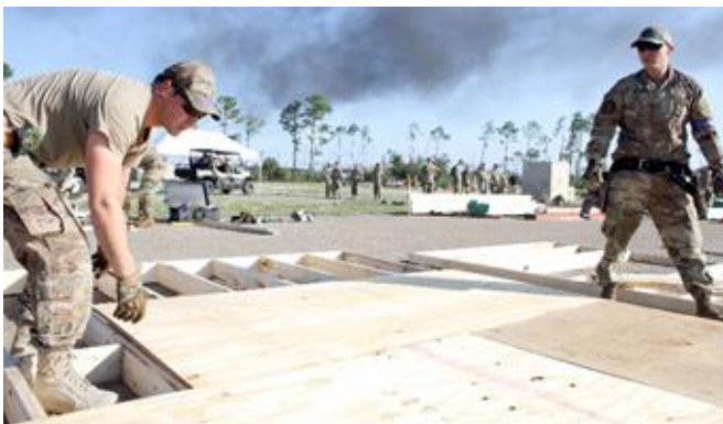
Participants from U.S. Space Force's 45th Civil Engineer Squadron, Patrick Space Force Base, Florida, begin the guard shack build event.
