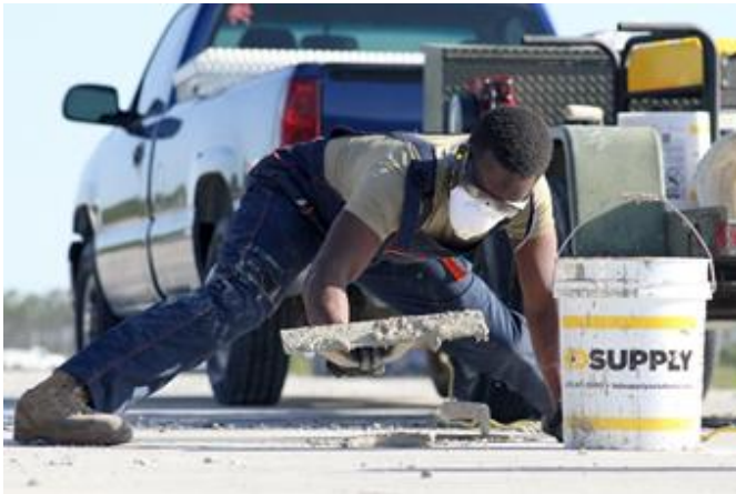
Participants from U.S. Air Forces in Europe's 31st Fighter Wing, Aviano Air Base, Italy, take part in the airfield spall repair event.
