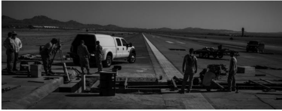
Airmen perform flight line maintenance. The construction occurred on both ends of the Nellis flight line and will make flying operations more efficient for the future.
