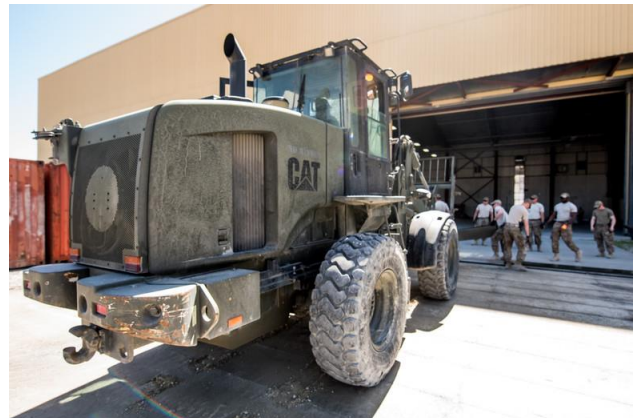
Airmen from the 1st Civil Engineer Group's 577th Expeditionary Prime Base Engineer Emergency Force Squadron do construction work on an F-16 maintenance hangar at Bagram Airfield, Afghanistan, May 4, 2018. Separate from traditional civil engineer units, the members of the 1st ECEG perform construction and repair in high-risk environments all across the area of operations.
