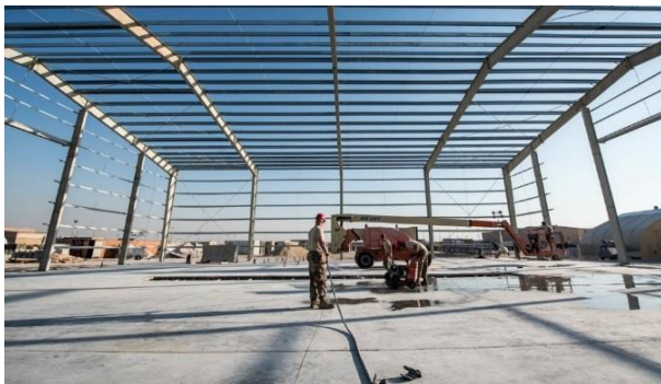
Airmen from the 557th ERHS work on a new structure that will house the 379th Expeditionary Logistics Readiness Squadron's vehicle maintenance at Al Udeid Air Base.
