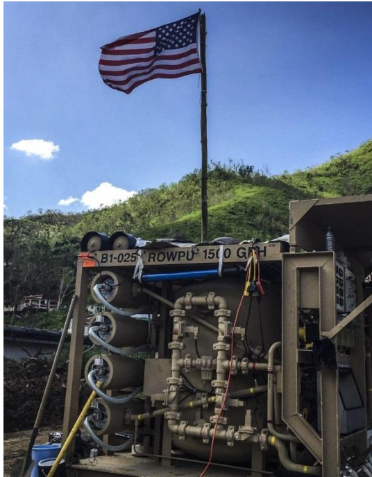
Photo shows a Reverse Osmosis Water Purification Unit (ROWPU) the Airmen from the 200th RED HORSE Squadron use to purify water in Comerio, Puerto Rico.
