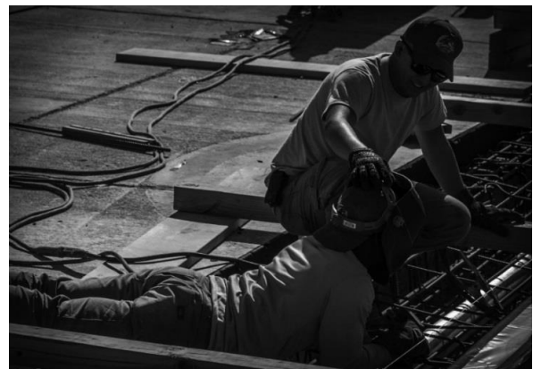
Airmen assigned to the 820th RED HORSE Squadron take a momentary break from welding rebar during flight line maintenance on Nellis Air Force Base, Nevada, Sept. 20, 2017. The Airmen of the 820th RHS finished this project in five months' time.
