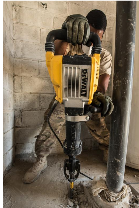
An Airman from the 1st Civil Engineer Group's 577th Expeditionary Prime Base Engineer Emergency Force Squadron does construction work on an F-16 maintenance hangar at Bagram Airfield, Afghanistan, May 4, 2018.
