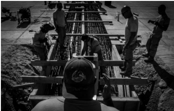
Airmen lay and weld rebar on a construction site on the flight line. Multiple squadrons assisted in the coordination of the construction including the 57th Operations Support Squadron and 99th Civil Engineer Squadron.
