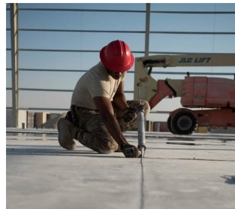
U.S. Air Force Staff Sgt. Forrest Dickson, a pavement and equipment journeyman seals concrete joints in the new structure.
