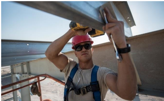
U.S. Air Force Senior Airman Bryan Smith, a structural journeyman assigned to the 557th Expeditionary Rapid Engineer Deployable Heavy Operational Repair Squadron Engineers (RED HORSE) Squadron, fastens bolts on to a new structure that will house the 557th ERHS vehicle maintenance at Al Udeid Air Base, Qatar. The 557th ERHS has over 200 Airman that specialize in jobs that include heavy equipment operators; heating, ventilation, air conditioning technicians; structures specialists; electricians and plumbers, deployed across the U.S. Central Command area of responsibility.
