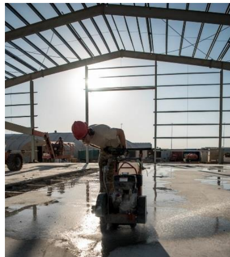
U.S. Air Force Airman 1st Class Charles Sage, a pavement and equipment journeyman assigned to the 557th ERHS, cuts concrete for joint in the new structure that will house the 557th ERHS vehicle maintenance.
