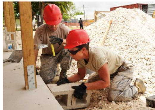
U.S. Air Force Staff Sgt. Natalie Taylor, right, heavy equipment operator for the 823rd RED HORSE Squadron, places a cinder block as a splash pad for a gutter down spout while U.S. Air Force Staff Sgt. Justin Jones, heavy equipment operator for the 823rd RED HORSE Squadron, ensures proper placement of the block at Ladyville Technical High School May 31, 2013.
