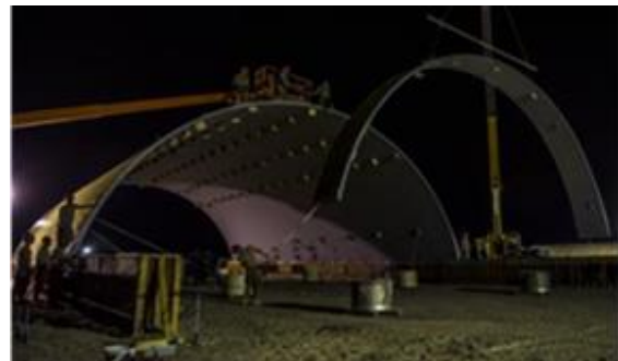
Airmen from the 557th Expeditionary RED HORSE Squadron use a crane to position steel arches for a K-Span building.
