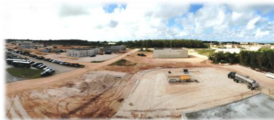
Constructing PACAF's new Regional Training Center, the 554 RHS used their "Can Do, Will Do" attitude to achieve mission success.
