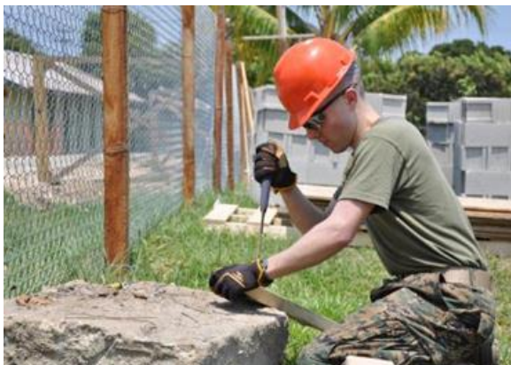
Marine Corps Lance Cpl. Erich Sullivan, combat engineer from Engineer Company Marine Wing Support Squadron 472, removes a nail from a piece of wood so it can be reutilized for the construction of Ladyville.
