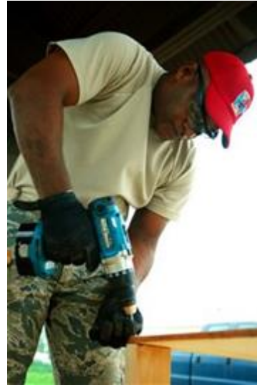
Master Sgt. Roberto Pitter drills a screw into an air conditioner deflector. Pitter and 13 other members from the squadron provide civil engineer support to Rush Park, an expeditionary-like community of temporary quarters for exercise augmentees.
