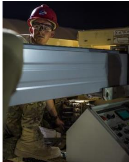
Staff Sgt. James Derbyshire, 557th Expeditionary RED HORSE Squadron structures craftsman, runs an Ultimate Building Machine to shape steel arches for a K-Span building Aug. 3, 2014.
