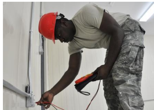
Tech. Sgt. Elisha Frazier, electrician from the 556th RED HORSE Squadron, tests the voltage at Ladyville Technical High School.
