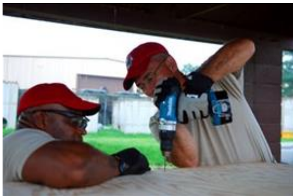
Master Sgt. Roberto Pitter and Tech. Sgt. Edward Mendiola, 254th RED HORSE squadron members, build an air conditioner deflector at Rush Park, Osan Air Base, South Korea, during the Ulchi Freedom Guardian exercise, Aug. 13, 2014. RED HORSE personnel helped create a home away from home for UFG participants.
