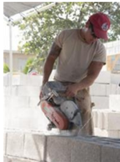
U.S. Air Force Senior Airman Justin Gonzalez, New Horizons pavements and construction equipment operator deployed from the 820th RED HORSE Squadron at Nellis Air Force Base, Nev., cuts blocks for use on the Sadie Vernon Technical High School construction site April 24, 2014, in Belize City, Belize.
