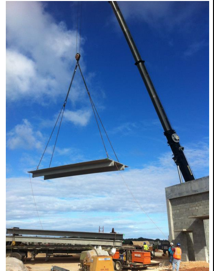
120-Ton Crane lifting a Double Tee beam to place on the building walls. The Tee beam construction was a new construction technique developed by 554th.
