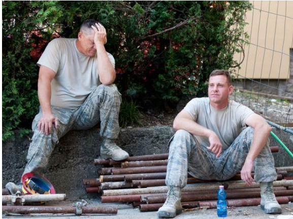
Master Sgt. Donald Maier, left, and Tech Sgt. Douglas Dial, of the 219th RED HORSE Squadron, take a work break after working at an elementary school in Ogulin, Croatia June 19.
