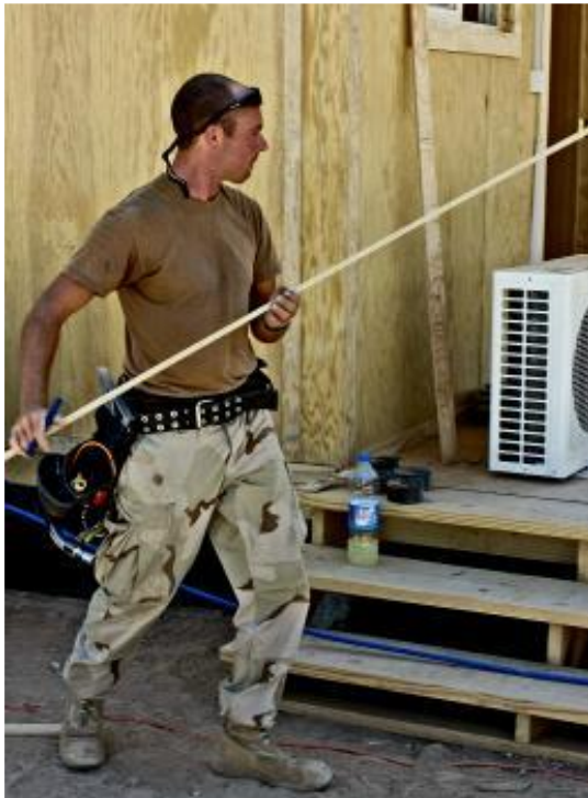
Staff Sgt. Josh Florea, Structural Engineer of Lincoln, Neb. is constructing one of 10 new housing units on Contingency Operating base Speicher.
