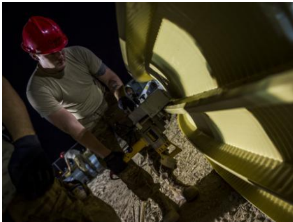
Senior Airman James Driscoll, 557th Expeditionary RED HORSE Squadron pavement and equipment operator, uses a hand seamer to bind two steel arches together.
