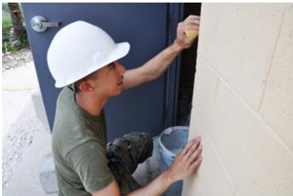
U.S. Marine Corps Sgt. Robert Lafleur, combat engineer from the Marine Wing Support Squadron 472, cleans excess caulk from the door frame at Ladyville.
