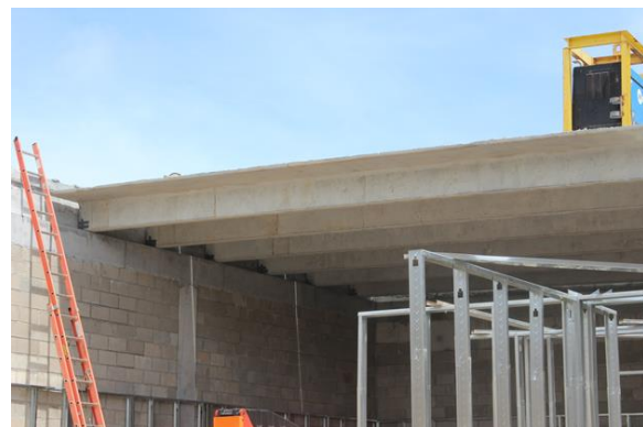
With no need for temporary supports, interior framing started prior to Double Tee installation.
