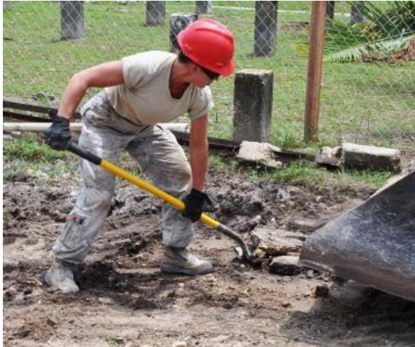
U. S. Air Force Staff Sgt. Natalie Taylor, heavy equipment operator from the 823rd RED HORSE Squadron, shovels dirt and rock in order to clear and level the ground at Ladyville.
