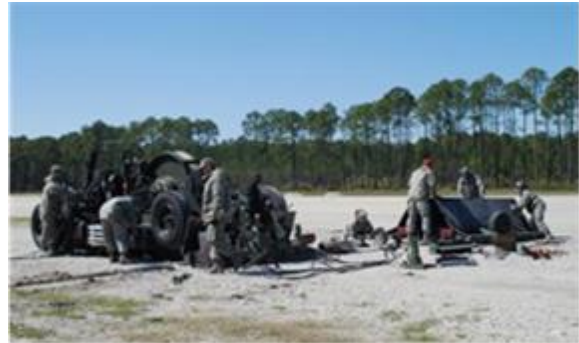
Civil Engineers of the 181st Intelligence Wing, under the supervision of Silver Flag cadre, assemble the Mobile Aircraft Arresting System (MAAS) during Exercise Silver Flag, Tyndall Air Force Base, Fla., March 26, 2013. The MAAS is a cabling system used to stop an aircraft that has lost braking power for landing.
