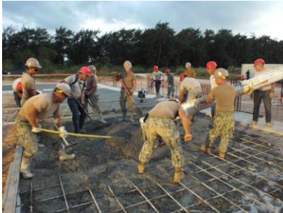
Navy Seabees and RED HORSE Airmen working together to place the foundation of a new PRTC Silver Flag building.
