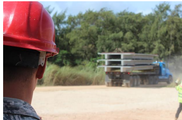
A 554 RHS Airman watches as Double Tee beams are delivered to the job site.
