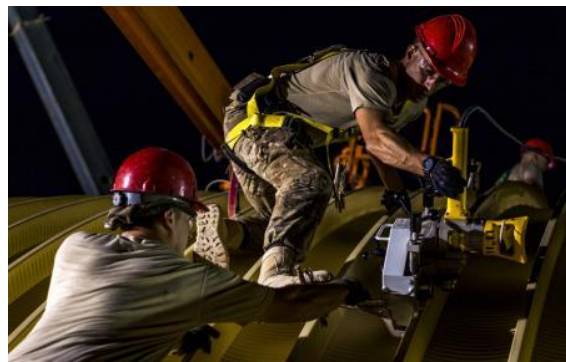
Senior Airman Nathan Hagy 557th Expeditionary RED HORSE Squadron water fuels systems maintenance journeyman, passes a hand seamer to Staff Sgt. Nicholas Mundorff, 557th ERHS, while binding two steel arches together.
