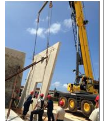
Future construction plans will use the Tilt-up design with the new double T-Beams for the roof systems which will save money and decrease construction time.
