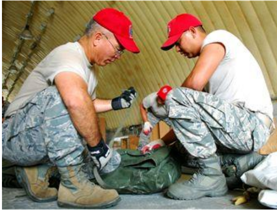
Tech. Sgt. Edward Mendiola and Senior Airman Jamie Torres, 254th RED HORSE members, fasten TEMPER tents for storage at Rush Park. RED HORSE staff traveled from Andersen Air Base, Guam, to provide civil engineer support during the exercise.
