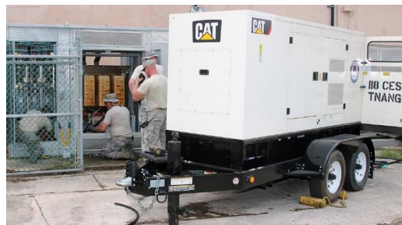
Airmen of the 118th Prime Power flight, work on a generator at Muniz Air National Guard Base, Puerto Rico, Oct. 11.
