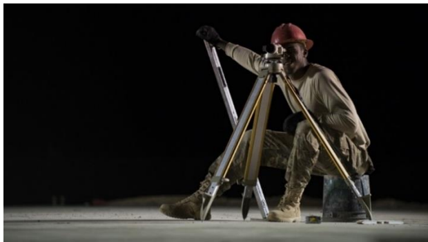
Staff Sgt. Jackie Timmons, structural craftsman, adjusts a laser level to ensure construction is started on the proper elevation June 27, 2017, in Southwest Asia.
