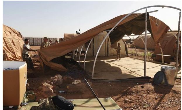
Airmen from the 724th Expeditionary Air Base Squadron take down tents from the old base to move to a new location.
