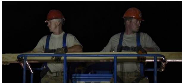
Tech. Sgt. Derek Miller, heating ventilation air conditioning craftsman, left, and Staff Sgt. Shannon Beavin structural craftsman, set up the structural frame of a building face.
