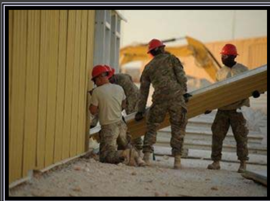
SOUTHWEST ASIA – Airmen from the 557th Expeditionary RED HORSE Squadron attach walls to the frame of a new RED HORSE facility here Dec. 27, 2011. The facility is the new home of the 1st Expeditionary RED HORSE Group, which oversees all Air Force construction operations throughout Southwest Asia. RED HORSE stands for Rapid Engineer Deployable, Heavy Operations Repair Squadrons, Engineer. (U.S. Air Force photo/Staff Sgt. Nathanael Callon)
