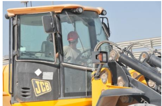
Staff Sgt. Jennifer Cowhick, 557th Rapid Engineer Deployable Heavy Operational Repair Squadron Engineer/Heavy Equipment Operator, using the hydraulic hammer to excavate the old concrete to make the new taxiway wider Jan. 30 at Al Udeid Air Base, Qatar.
