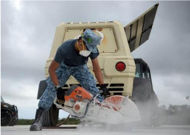
Republic of Singapore Air Force Military Expert 2 Wei Han Tan, a crater repair instructor, uses a pavement saw while repairing chips in an airfield during Partner Nation Silver Flag.
