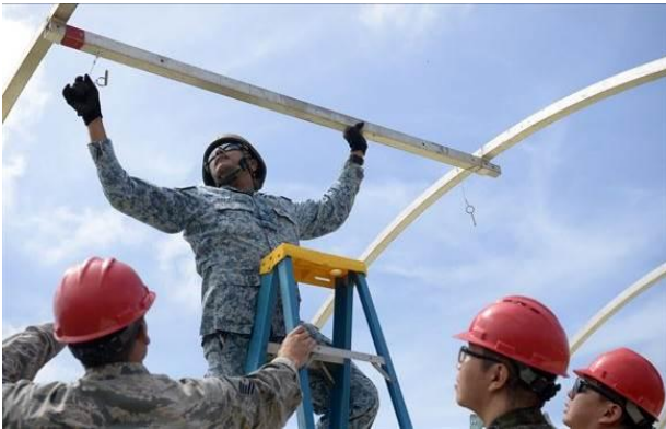
Republic of Singapore Air Force Military Expert 6 Nagenthiran Thurairaj, a 508th Engineer Squadron commanding officer, assembles a frame for a small shelter system during Partner Nation Silver Flag.
