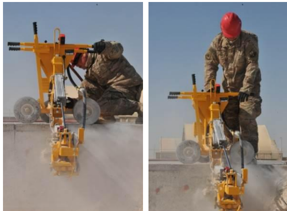
Senior Airman Shawn Polk, 557th Rapid Engineer Deployable Heavy Operational Repair Squadron Engineer/Heavy Equipment Operator, operates an E-Z Drill to drill holes for dowel placement Jan. 30 at Al Udeid Air Base, Qatar.
