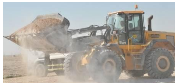
Staff Sgt. Jennifer Cowhick drives the front end loader to move base course.
