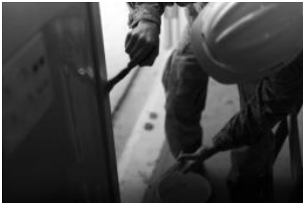
A 101st Civil Engineer troop paints door trim as part of a deployment for training.
