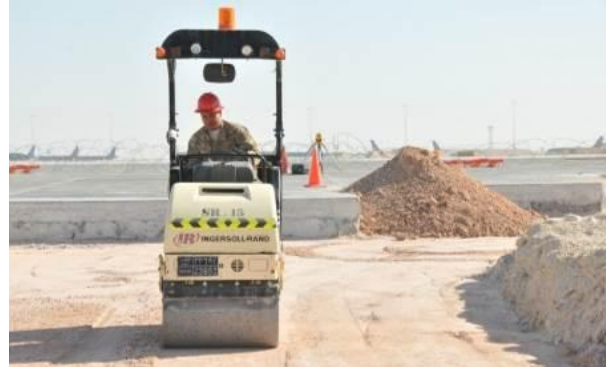
Staff Sgt. Edward San Nicolas, 557th Rapid Engineer Deployable Heavy Operational Repair Squadron Engineer Heavy Equipment Operator, drives a roller to compact the base course.
