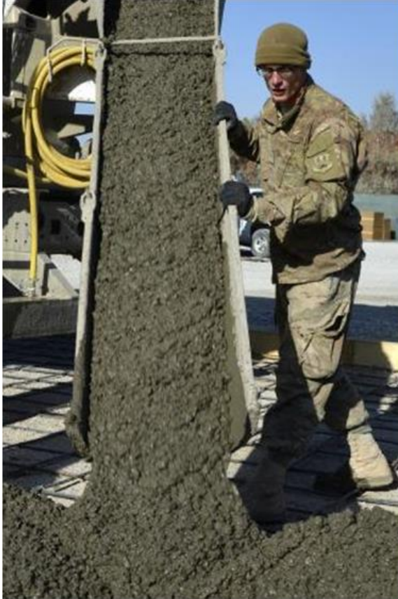
U.S. Air Force Airman 1st Class Austen Windle, 577th Expeditionary Prime BEEF Squadron pavements and equipment operator, helps with pouring the concrete foundation at Kandahar.
