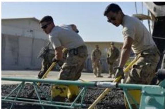
U.S. Air Force Senior Airman Dylan Sheets, 577th Expeditionary Prime BEEF Squadron heating, ventilation, and air conditioning, and Senior Airman Mervin Santa Maria, 577th EPBS electrician, rake concrete foundation at Kandahar. EPBS poured concrete for a large-area maintenance facility, which is about 8,000 square feet.
