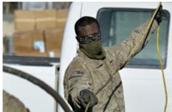
U.S. Air Force Senior Airman Andrew Wright, 577th Expeditionary Prime BEEF Squadron electrician, assists with pouring the concrete foundation.
