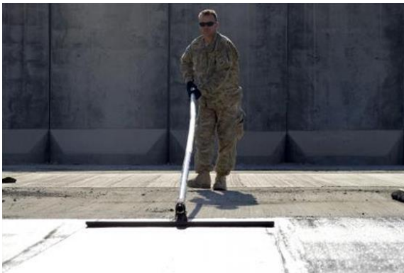
U.S. Air Force Staff Sgt. John Scherstuhl, 577th Expeditionary Prime BEEF Squadron pavements and equipment operator, smooths the concrete foundation.
