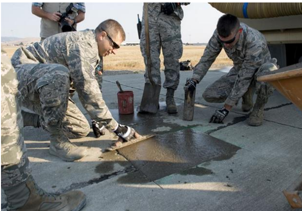
Airmen assigned to the 60th Air Mobility Wing complete a concrete taxiway repair at Travis Air Force Base, Calif., Aug. 19, 2016. 1st Expeditionary Civil Engineer Group airmen recently used similar techniques on a much larger scale to repair damage caused by Islamic State of Iraq and the Levant terrorists at Qayyarah West Airbase in
