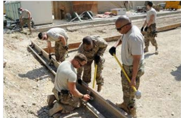
Members of the 577th Expeditionary Prime Base Engineer Emergency Force Squadron assemble a perimeter mold for a concrete pad on Bagram Airfield, Afghanistan, May 6, 2013. (All photos this article by U.S. Air Force photo/Staff Sgt. David Dobrydney)
