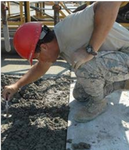
U.S. Air Force Staff Sgt. Christopher Lange, engineering technician, performs a concrete slump test during training. The slump test is used to ensure uniformity between individual batches of concrete.
