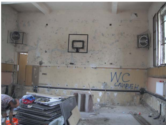
The VII Middle School before renovation. Work included new flooring, new plaster on the walls, new lights, cages around windows and lights,
