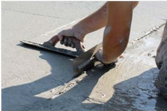
An airman smoothing and edging concrete during training. (All photos by U.S. Air Force photo by Airman 1st Class Brittain Crolley)
