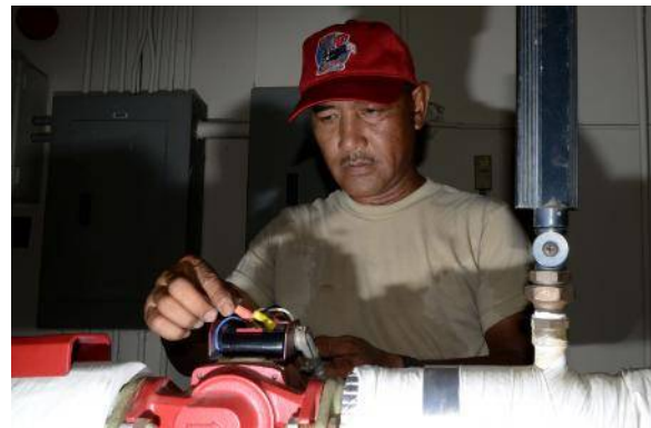
U.S. Air Force Staff Sgt. Edward Fernandez, 254th RED HORSE Squadron structure craftsman, troubleshoots a plumbing unit at Rush Park, Osan Air Base, Republic of Korea, during the Ulchi Freedom Guardian 2013 exercise, Aug. 18, 2013. The 254th RHS has been preparing and supporting the UFG since 2006 ensuring participants have essential water, heat and electrical power generation. UFG is an annual training, defense-oriented exercise developed around realistic scenarios designed to defend the ROK, protect the region, and maintain stability on the Korean Peninsula. (U.S. Air Force photo/Staff Sgt. Sheila deVera).
