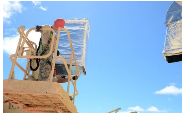
Tech. Sgt. Lonnie Battenfield, left, 556th RED HORSE Squadron utilities craftsman, and Staff Sgt. Mathew Scroggins, 556th RHS operations management technician, transport an exterior duct section to the warehouse.
