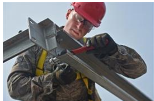
Pennsylvania Air National Guard Senior Airman Daniel Clark, 201st RED HORSE structures technician, tightens a bolt on a purlin beam as part of the construction process for the new medical clinic. The bolts that secure the purlin beam to the trusses are tightened using locking washers to keep them from loosening under stress.
