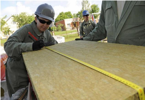
Staff Sgt. Amanda Turnwald, 127th Civil Engineering Squadron engineering assistant, marks a measurement on a piece of rock wool insulation at the kindergarten.
