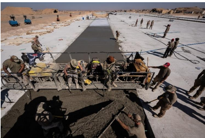
1 st ECEG Pavements and Heavy Equipment Operators place, finish, and burlap a new lane. The 1 st ECES is placing a total of 12,000 cubic meters throughout the entire project. This single pour is 340 cubic meters.
