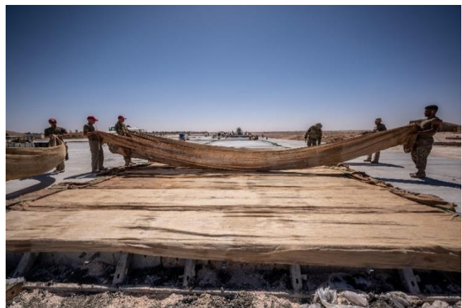
1 st ECEG Airmen place burlap on top of finished concrete. Damp burlap cloth is placed on freshly poured concrete and is continuously hosed down to ensure the concrete is hydrated during the curing process.
