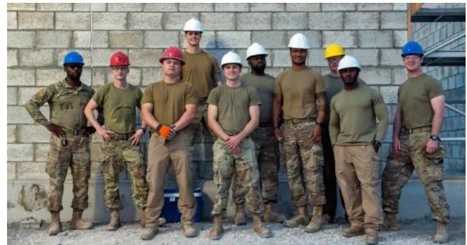
Members of the U.S. Air Force 1 st ECEG pose for a group photo on a construction site on Al Udeid Air Base, Qatar, June 15, 2022. The group has been constructing a hardened latrine, shower and laundry facility for the past three months.
