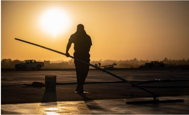
Technical Sgt. Nolan Denson, 1 st ECEG pavements and construction equipment operator craftsman, uses a bull float in the finishing process of a concrete pour. Bull floating helps level the concrete, making it easier to apply a non-skid finish at the end.
