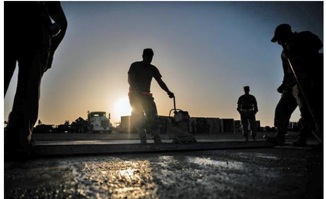
Senior Airman Alexander Curtiss, 332 nd ECES structural specialist journeyman, uses a power concrete screed to confirm a level surface.
