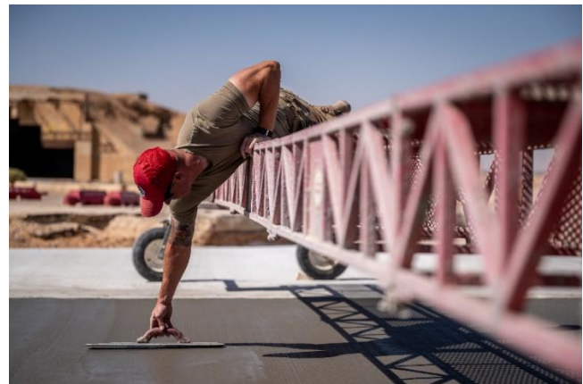
Tech. Sgt. James Gasbarro, 1 st ECEG project manager, stretches out from a platform to fix an abnormality in the concrete. Gasbarro is one of four project managers to oversee the overrun project that began in December of 2021.
