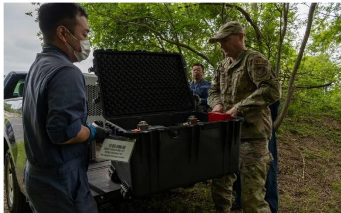
Members from the 35 th CES water and fuel system unload the WaFERS during setup. The system enables expedient or semi-permanent repair of mission essential water and fuel distribution lines and storage systems that support airbase resiliency.
