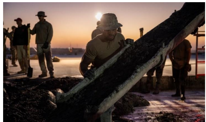
Staff Sgt. Devyous Barlow, 1 st ECEG lead chute operator, spreads concrete from a cement truck during a runway overrun repair project. Evenly spread concrete aids in preventing major high or low spots during the pour.
