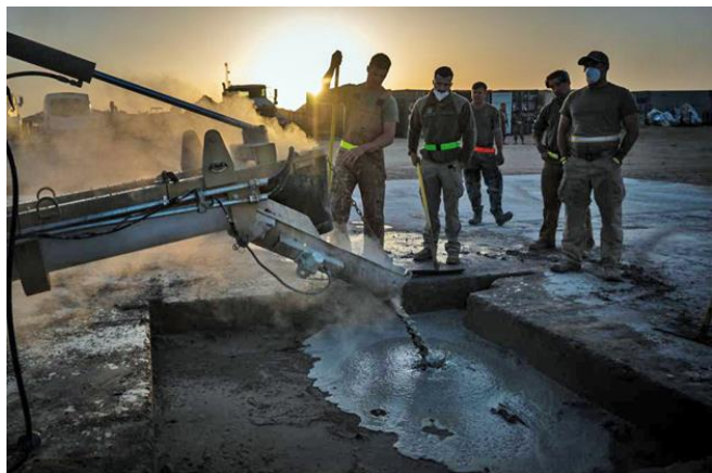
332 nd ECES Airmen pour water and quick-dry cement into a portion of damaged runway.
