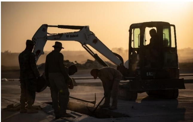
1 st ECEG Airmen remove wood forms used for airfield lighting placement. The runway extension, or overrun, will better accommodate aircraft take-off and landing operations and provide extended mission capabilities for the 332 nd AEW by replacing the non-load-bearing surface and providing improved capabilities in the event of an emergency takeoff or landing.
