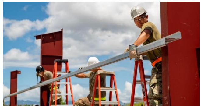
U.S. Air Force Staff Sgt Sittikai Wisanu, a heating, ventilation and air conditioning troop assigned to the 163 rd CES, works alongside fellow service members getting ready to pour concrete for the Training Facility foundation.
