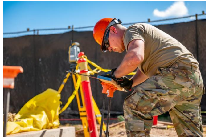
U.S. Air Force Senior Airman. Salvador Marroquin, a structures troop assigned to the 163 rd CES cuts forms for exterior doors near the Special Olympics Training Facility construction grounds on August 2, 2022.
