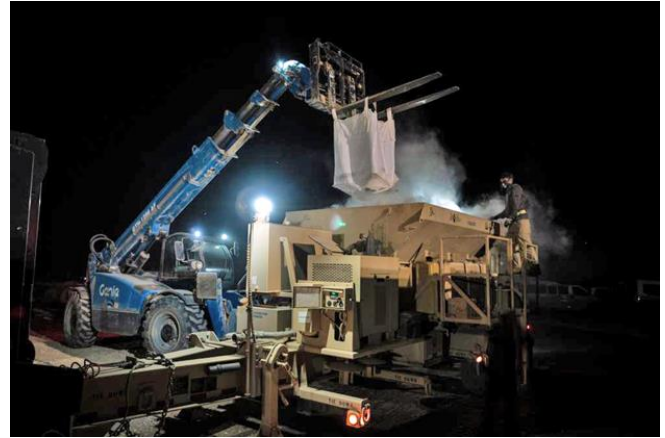
332 nd ECES Squadron Airmen expedite the repair of spalls with rapid-setting cement mix by emptying a bag of dry concrete into a mixer.
