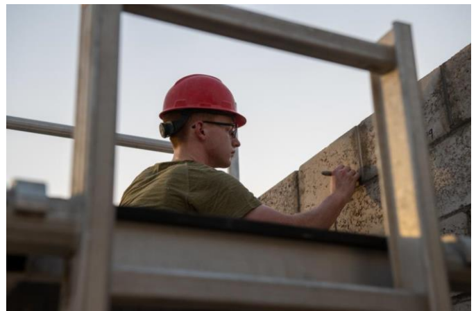
U.S. Air Force Senior Airman Ethan King, a structural journeyman with the 1 st ECEG, marks a wall for the placement of rebar. Rebar is placed within the masonry bricks, which are then filled with concrete in order to fully reinforce the structure.
