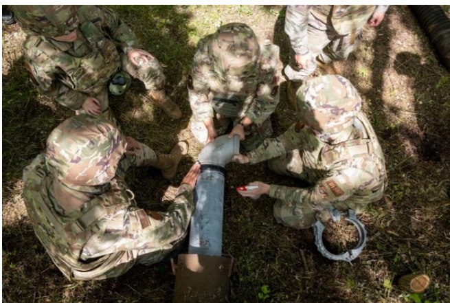
U.S. Airmen assigned to the 35 th CES water and fuel system set up the connection for a new water pipe. The 35 th CES Water and Fuels Systems Maintenance is responsible for the upkeep of Misawa’s water, sewer, and gas lines as well as all facilities with water and fuel infrastructure.
