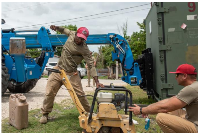
Senior Airman Emmanuel Herring, left, and Staff Sgt. Job Stark, right, pull start a compactor June 14, 2022 at the Ixlu Health Clinic in Guatemala. RS 22 serves to train U.S. civil engineers, medical professionals and support personnel while providing humanitarian assistance and joint training with partner.
