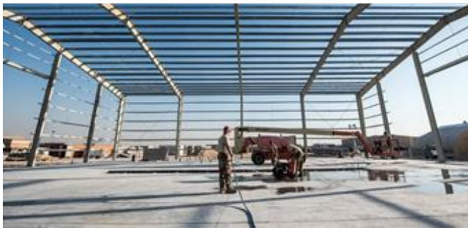
Airmen from the 557th “Red Horse” squadron build a structure at Al Udeid Air Base, Qatar, in 2017. (Phil Speck/U.S. Air National Guard).
