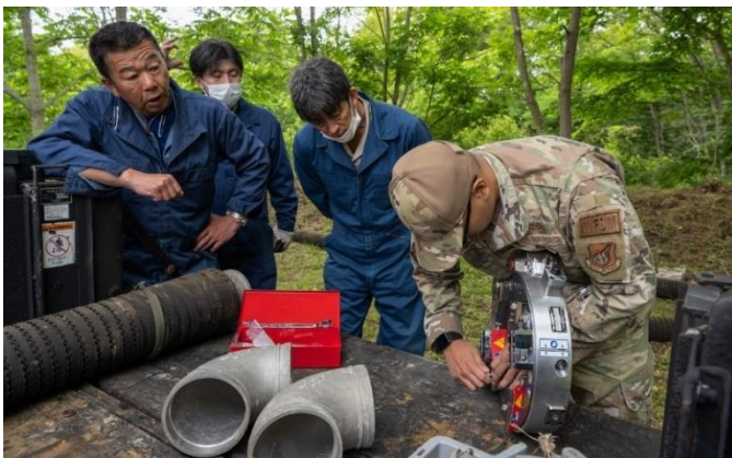
U.S. Air Force Senior Airman Joshua Sanchez, 35 th CES water and fuel system journeyman, puts together the new WaFERS during setup for the annual Prime BEEF. The process is used to fix damaged pipes to support rapid projection and application of U.S. military power, ensuring continuation of operations and installations around the globe.
