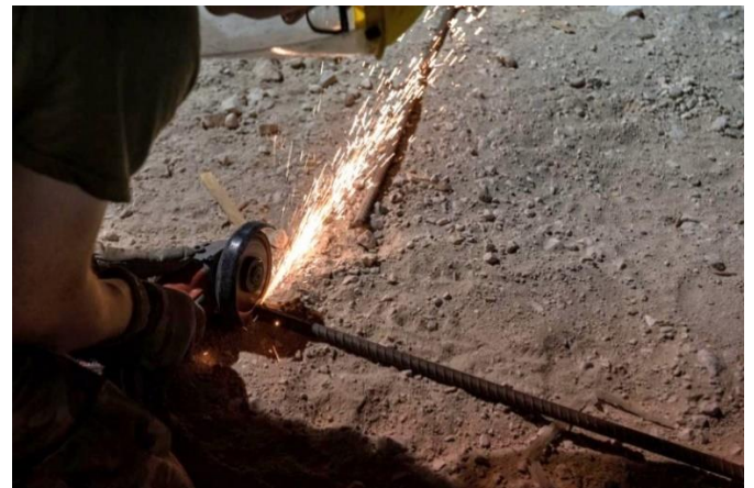
U.S. Air Force Senior Airman Ethan King, a civil engineer with the 1 st ECEG, cuts rebar during the construction project. Rebar is used to reinforce concrete when constructing buildings.
