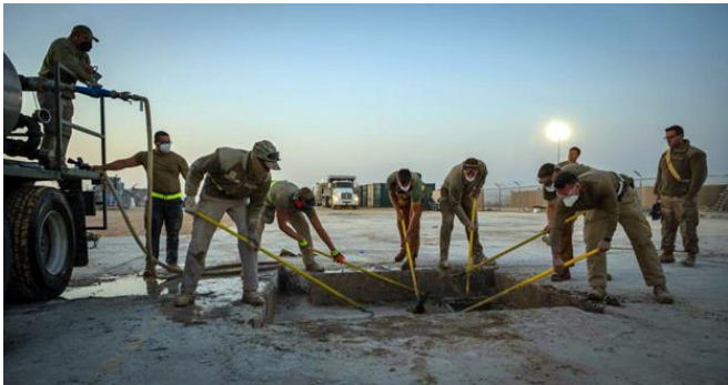
332 nd ECES Airmen mix water and a quick-dry filler to repair runway damage.
