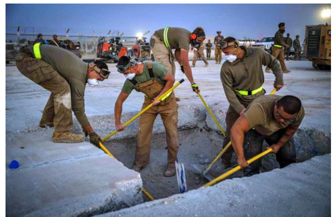
332 nd ECES Airmen measure the base of a crater to confirm it is at proper elevation before backfill material is placed within it.
