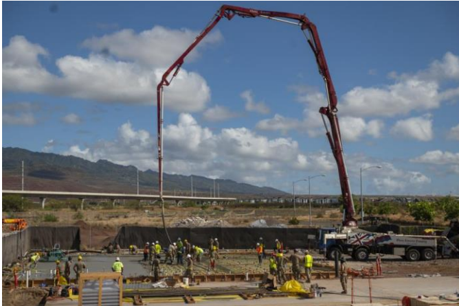
U.S. Air Force Airmen assigned to the 163 rd CES, work alongside local contractors to pour the concrete.
