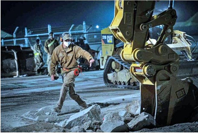
Technical Sgt. David McCoy, 332 nd ECES non-commissioned officer in charge of airfield pavements and logistics, gives spotting instructions to an excavator operator to remove debris and prepare a crater for backfill material.
