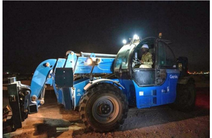
U.S. Air Force Tech. Sgt. Van Johnson, a structural journeyman with the 1 st ECEG, removes wooden pallets from a construction site as part of keeping the job site safe.
