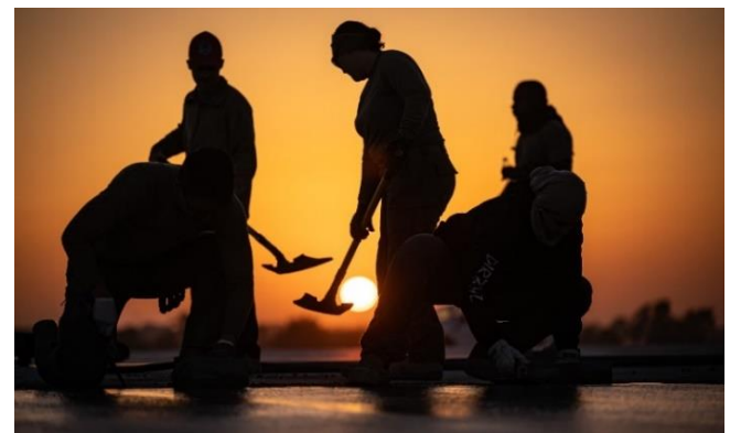
Staff Sgt. Glenn Scott and Staff Sgt. Tara Schnider, 1 st ECEG pavements and construction equipment operator craftsmen, edge concrete. Edging concrete produces a clean finish and helps resist chipping and spalling damage after forms are removed and joints are cut in.
