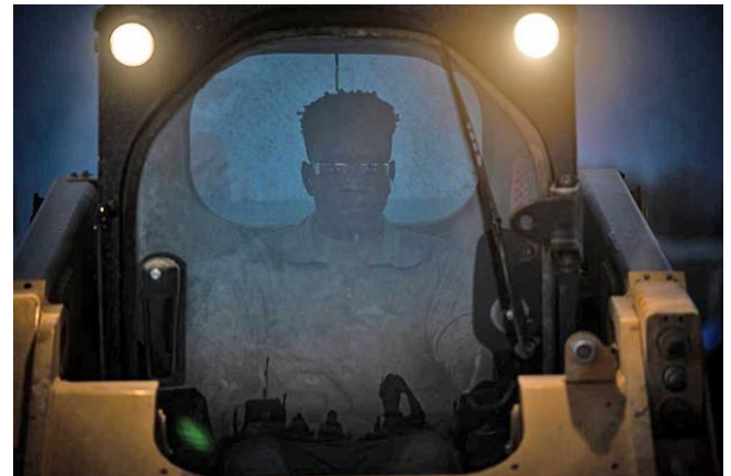
Staff Sgt. Kweku Awuah, 332 nd ECES water and fuel systems maintenance craftsman, operates a multi-terrain loader to clear debris after a simulated attack on a replicated runway.
