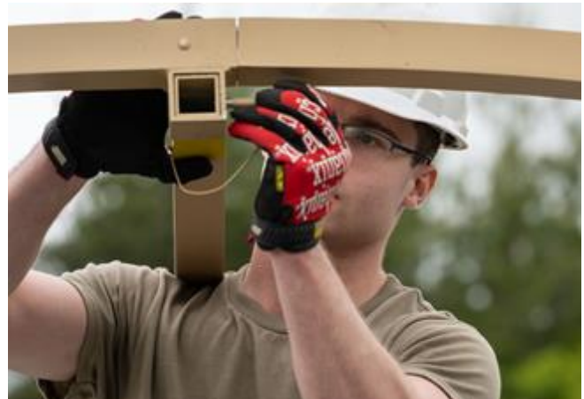
U.S. Airman 1st Class Ryan Gray, 35th Civil Engineer Squadron structures journeyman, places a pin to connect and lock a Disaster Relief Beddown System tent during the annual Prime BEEF training event.
