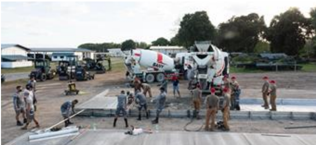
Airmen from the 819th RED HORSE Squadron out of Malmstrom Air Force Base, Montana, assist the Philippine Air Force in pouring concrete as part of a Field Training Event at Basa Air Base, Philippines, January 25, 2023.
