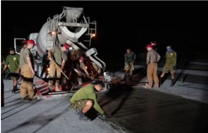
Airmen from the 819th RED HORSE Squadron assist Philippine Air Force Airmen in pouring concrete as part of the Field Training Event.
