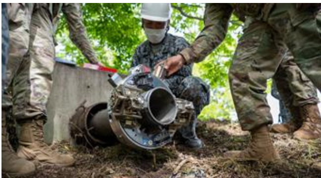
The 35th CES completes 2022 Prime BEEF training: Japan Air Self-Defense Force Tech. Sgt. Akashi Kikuchi, 3rd Air Wing Civil Engineer Squadron water and fuel system maintainer, looks at new components on the Water and Fuel Expedient Repair System during the annual Prime BEEF training at Misawa Air Base, Japan, June 14, 2022.
