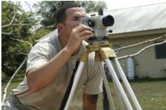
Staff Sgt. Joel Bradley, engineering assistant for the 823rd Red Horse Squadron, sets an auto level to check the final grade elevation at the construction site of the future Crooked Tree Government Primary School March 23, 2013. Civil engineers from both the U.S. and Belize will construct various structures at schools throughout Belize as part of an exercise called New Horizons. (U.S. Air Force photo and article by Master Sgt. James Law)
