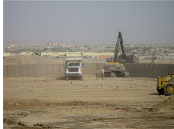
CAMP JOHN PRATT, Afghanistan – Airmen from the 554th RED HORSE Squadron use heavy machinery to fill up Hesco barriers with dirt to create the inner structure of a safety berm to surround and protect a fuel reservoir at Camp John Pratt, Afghanistan, in October 2012. The 554 RHS is currently deployed downrange in support of U.S. Central Command's Operation Enduring Freedom. (Courtesy photo)
