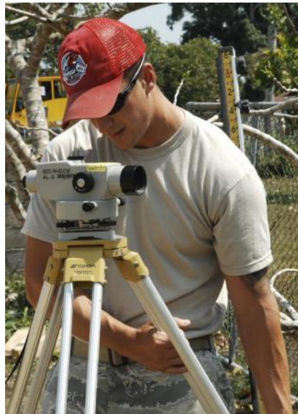
Staff Sgt. Joel Bradley, engineering assistant for the 823rd Red Horse Squadron, ensures an auto level is level while setting it up for a final grade elevation check March 23, 2013, at the construction site of the future Crooked Tree
