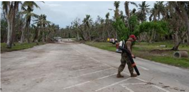
U.S. Air Force Master Sgt. Raymon Charron, 560th RED HORSE, Joint Base Charleston, South Carolina, pavements and equipment noncommissioned officer in charge, uses a backpack air blower on remaining debris.
