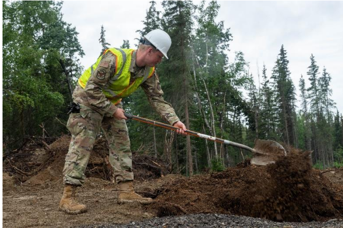
Senior Airman Nathan Smith, a 934th Airlift Wing Civil Engineering Squadron engineering journeyman, backfills a trench.
