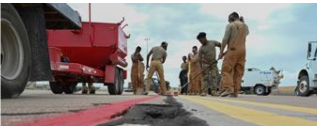
Airmen from the 49th Civil Engineer Squadron perform airway pavement repair. The 49th CES pavement and construction Airmen are often referred to as “Dirt Boyz” for their constant interaction with various heavy construction equipment and hand tools used to repair and maintain Holloman’s roads, airfields, fences and drainage systems.
