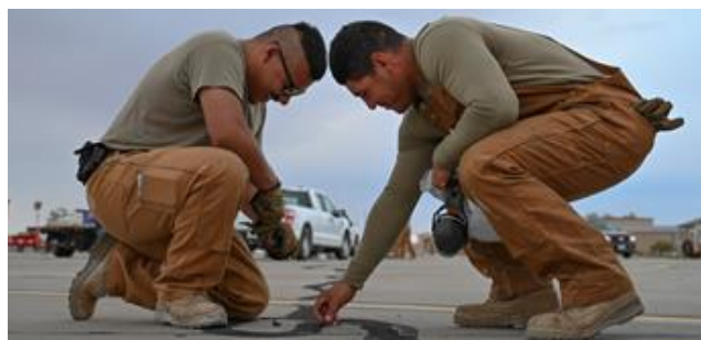
U.S. Air Force Airman 1st Class Aaron Escoto, left, and U.S. Air Force Airman 1st Class Jorge Capistran, 49th Civil Engineer Squadron pavement and construction equipment journeymen, inspect sealant installed during a previous pavement repair at Holloman Air Force Base.
