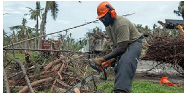
U.S. Air Force Staff Sgt. Kevin Vincent, 567th RED HORSE Engineer, Seymour Johnson, North Carolina, pavements and equipment journeyman, uses a chainsaw to cut tree branches.
