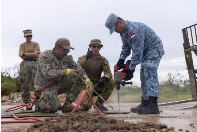
Navy Seabees work alongside Royal Australian Air Force and Republic of Singapore Air Force Airmen for the airfield damage repair exercise.
