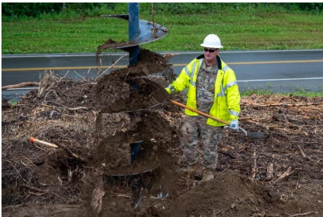
Tech Sgt. Andrew Brinza, a 934th Airlift Wing Civil Engineering Squadron structures craftsman, removes the dirt off of heavy machinery during the upgrade of Camp Mad Bull’s electrical system at Joint Base Elmendorf-Richardson, Alaska, on Aug. 9, 2023.
