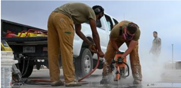
U.S. Air Force Senior Airman Jacquetz Craddieth, left, and Senior Airman Eric Wheeler, 49th Civil Engineer Squadron pavement and construction equipment journeymen, utilize a K-12 concrete saw to repair a runway at Holloman Air Force Base.
