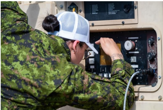
Royal Canadian Air Force Aviator Marissa Browning, 4 Mission Support Squadron electrical generation systems technician, participates in a power unit operations event April 23. (U.S. Space Force photo by Airman 1st Class Spencer Contreras).
