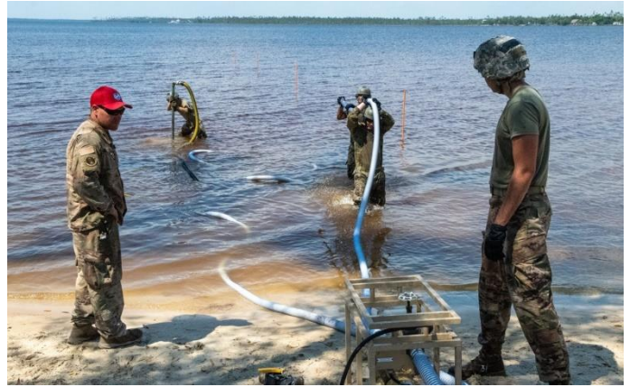
A member of the 801st RED HORSE Training Squadron evaluates members of the Air Force Reserve Command Civil Engineer team, led by the 482nd Civil Engineer Squadron from Homestead Air Reserve Base, Florida, as they work together during a water purification exercise, April 25. (U.S. Air Force photo by Armando Perez).
