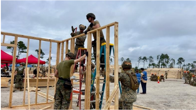
Members of the U.S. Marine Corps Civil Engineer team, led by the 172 Marine Wing Support Squadron from Okinawa, Japan, participate in a security guard shack exercise at Readiness Challenge X in Tyndall Air Force Base, Florida, April 21, 2024 (U.S. Air Force photo by Armando Perez).
