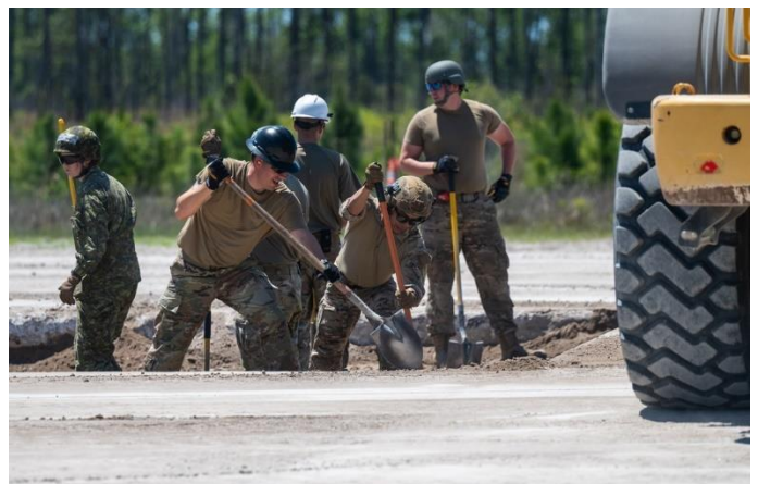
Members of the Coalition Team dig during an airfield damage repair event April 23. (U.S. Space Force photo by Airman 1st Class Spencer Contreras).
