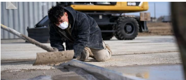
U.S. Air Force Senior Airman Omar Becerra, 51st Civil Engineer Squadron pavement and construction heavy equipment operator, removes excess concrete during ROAR training. Airmen tested a flowable fill concrete cap over crushed stone to evaluate whether the streamlined method can improve repair timelines during simulated attack scenarios.
