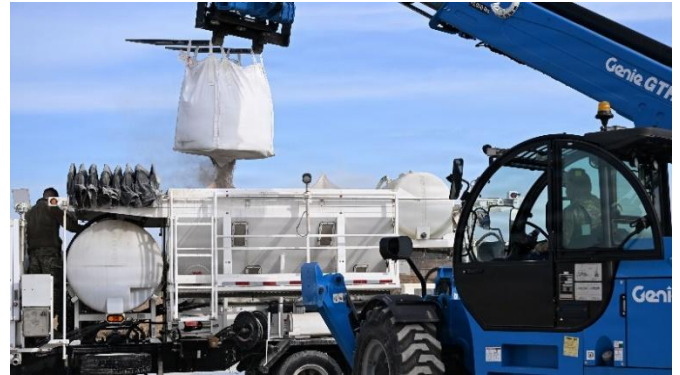
Airmen mix concrete powder and water in a volumetric mixer during ROAR training. The training evaluated ROAR, an installation-specific method focused on restoring minimum runway capability quickly during contingency operations.
