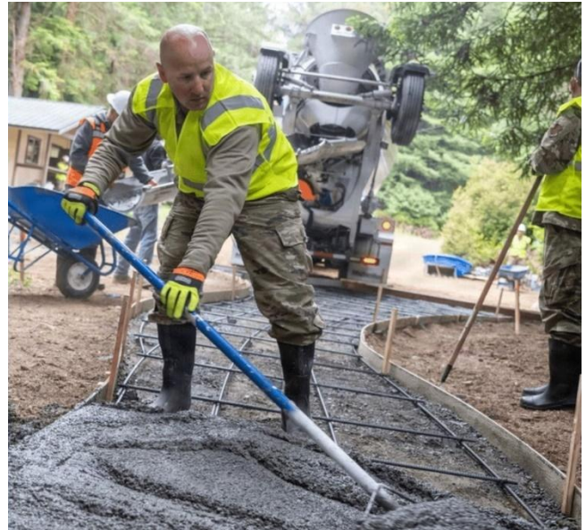
Airmen from the 124th Civil Engineer Squadron strengthened infrastructure at the Wolf Creek Education Center in Redwoods National Park, California, during an Innovative Readiness Training mission that balanced community support with mission-ready skill development. Through multi-trade construction and collaboration with park partners and tribal nations, the mission enhanced public facilities while building teamwork, leadership, and expeditionary readiness.
