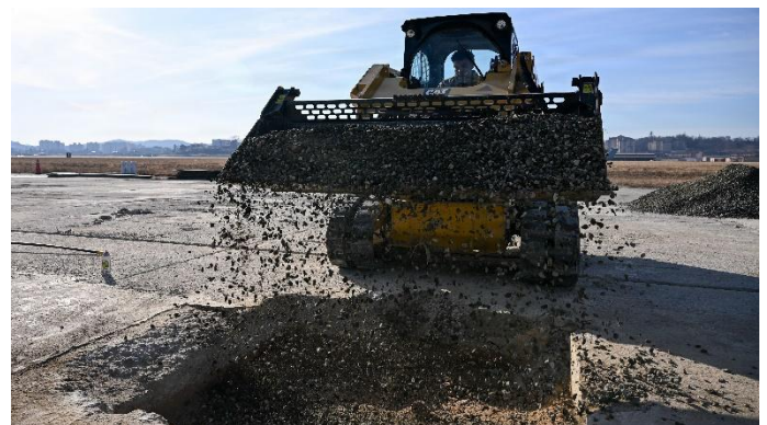
An Airman, dumps rocks into a crater. Airmen placed flowable fill concrete over compacted crushed stone as part of Osan's ROAR concept, designed to rapidly generate aircraft launch capability.
