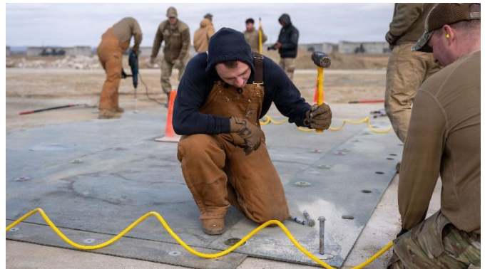
U.S. Air Force Senior Airman Elyjah James, 51st Civil Engineer Squadron structural journeyman, hammers down a screw during ROAR training at Osan Air Base, Republic of Korea, 27 February 2026. The Osan-developed recovery method prioritizes speed to achieve approximately 300 aircraft passes before transitioning to longer-term repair solutions.
