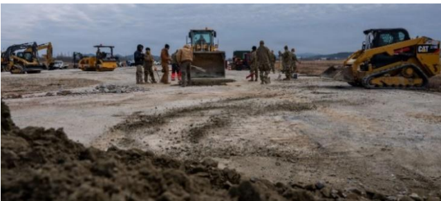
Airmen remove excess debris in preparation for fiber reinforced to be installed. The panel-based technique is designed to rapidly return the runway to operational status in support of aircraft launch operations.
