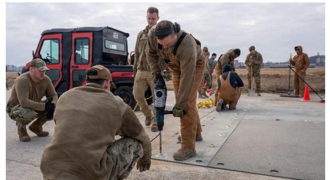
U.S. Air Force Airmen assigned to the 51st Civil Engineer Squadron drill concrete anchors. The fiber reinforced panels are used to quickly allow aircraft to takeoff in a contingency environment where the airfield may have been subject to damage.
