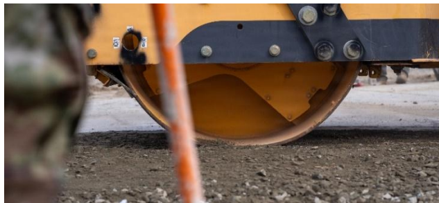
Airmen flatten compact crushed stone in preparation for fiber reinforced panels to be installed. ROAR focuses on quickly restoring limited airfield capability to sustain combat airpower while follow-on repairs are implemented.
