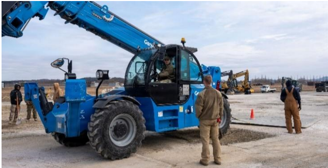
Airmen pull a fiber reinforced panel. The panel-based technique is designed to rapidly return the runway to operational status in support of aircraft launch operations.
